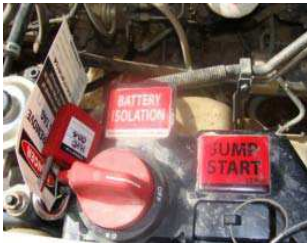
Light vehicle main isolator where fitted
